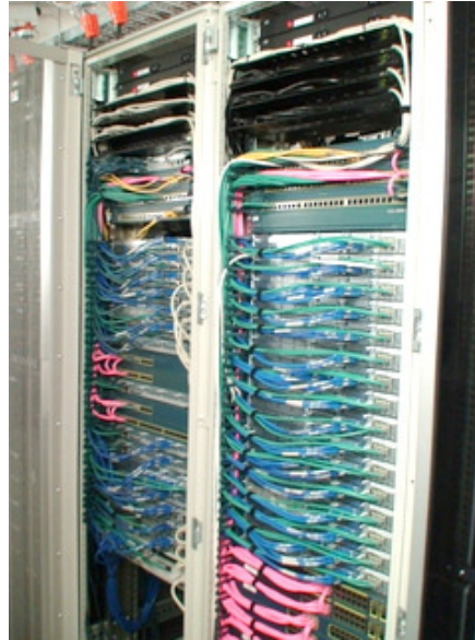
Figure 1 Netlab Servers and associated laboratory equipment
