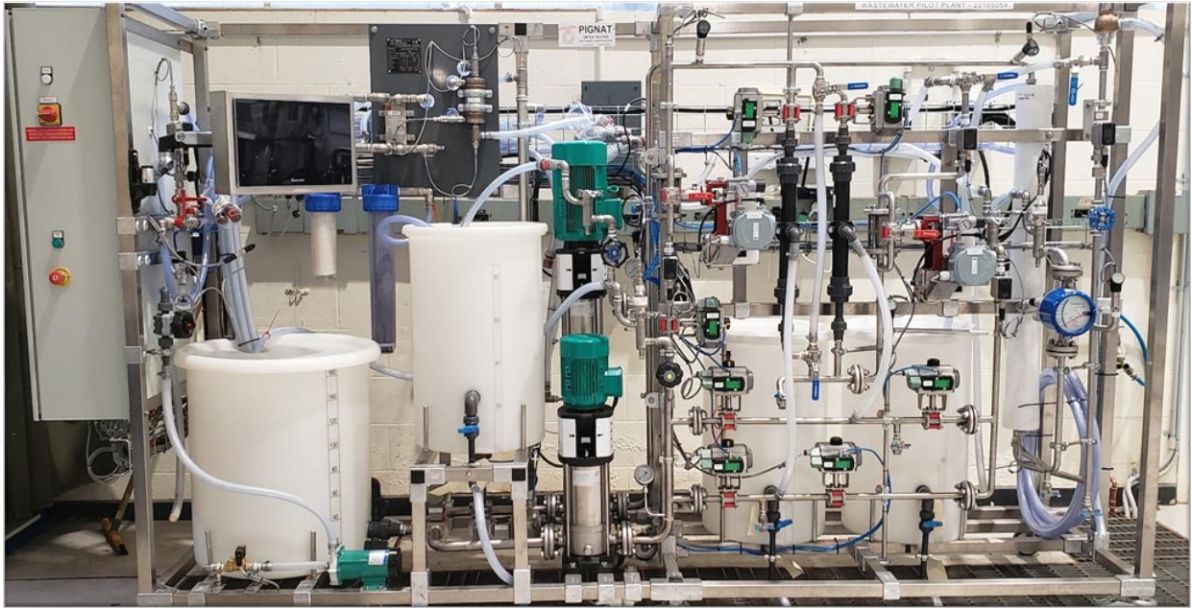
Figure 1: The Monash Membrane Pilot Plant
